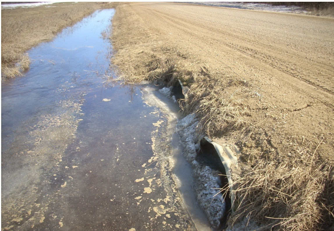
22 - Bear River North Drainage Line 1 @ RR12-2 - Twin 1600 Low Cover (April 2014) Page 11 of 49
