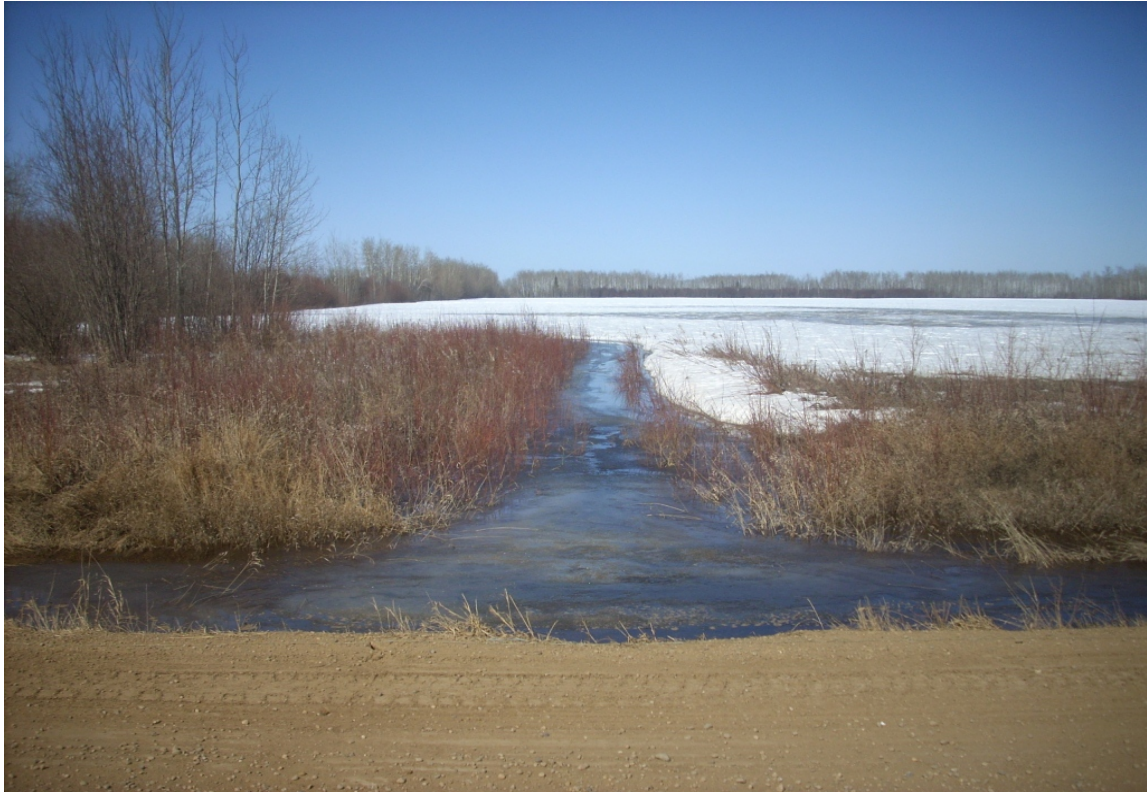
21 - Bear River North Drainage Line 1 @ RR12-2 - Twin 1600 CSP Inlet (April 2014)
