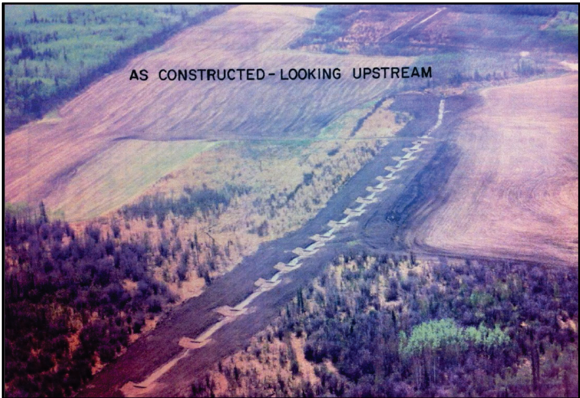
Figure 4-9 Photo of the completed Buffalo Head Prairie Flood Control Project – Line A1 (photo by Bekevich Engineering Ltd.).
