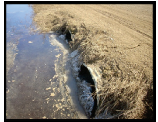
Figure 6-2 Culverts half full with ice (RR 122)
