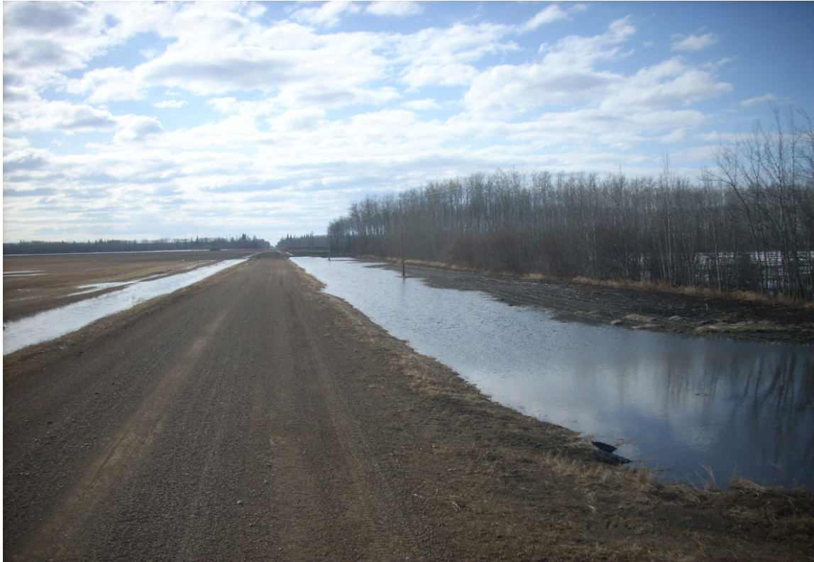
55 - TR 105-4 east of RR 14-0 - Looking West - Undersized CSP (April 2014)
