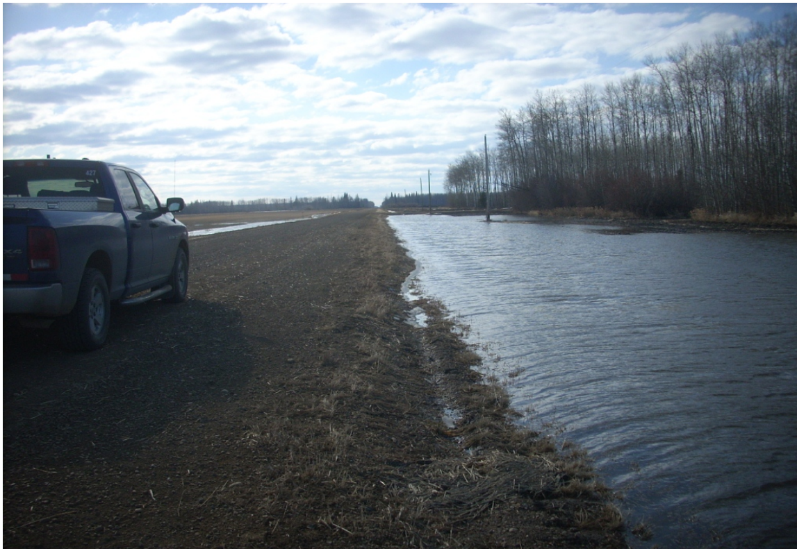
56 - TR 105-4 west of RR 14-0 - Ditch Full (April 2014)
