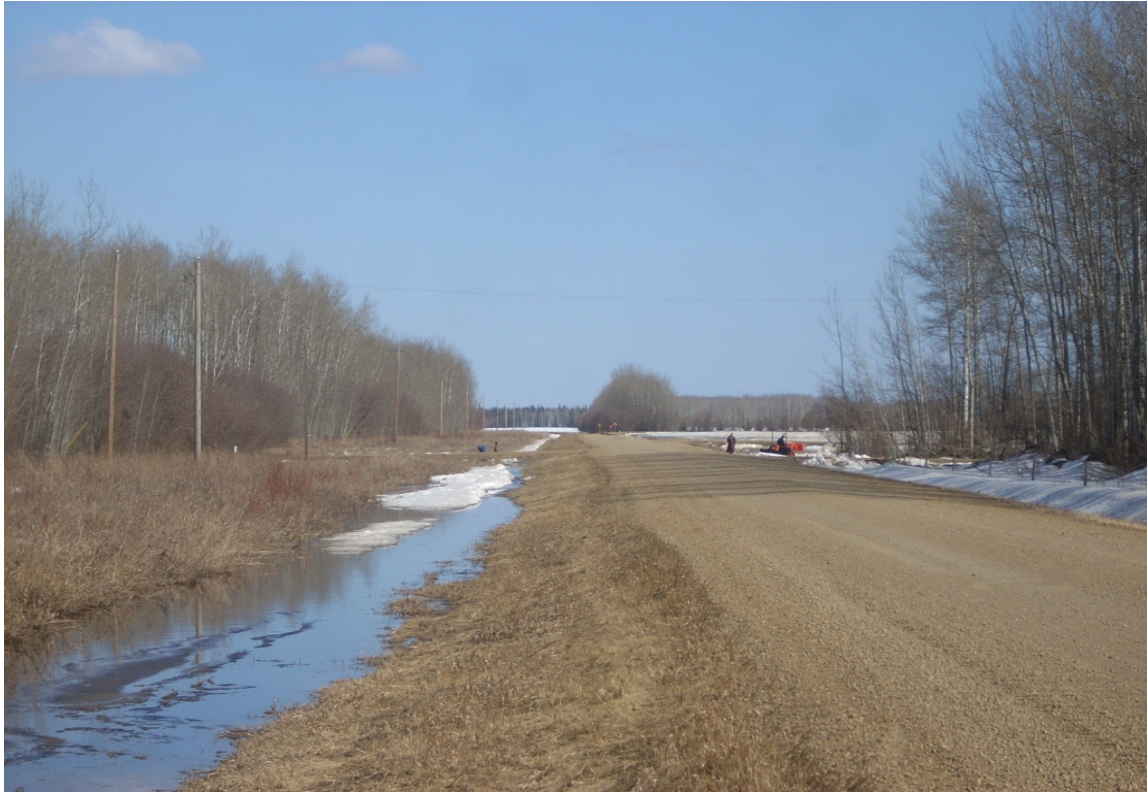
43 - TR 106-0 west of RR 13-4 - Looking East - Landowners Digging Out Culverts (April 2014)
