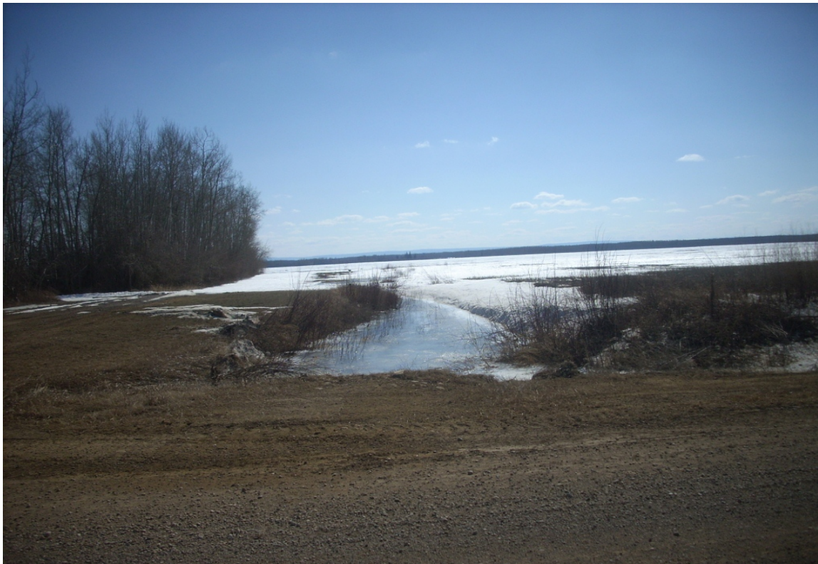
16 - Bear River North Drainage Line 1 @ TR 107-2 - South Culvert Invert (April 2014) Page 8 of 49
